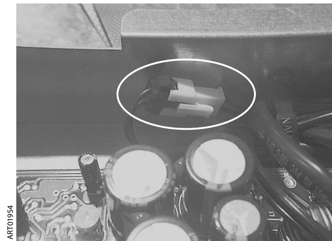
Figure 7. Evaporator Thermistor Connection (Inside Power Supply)
